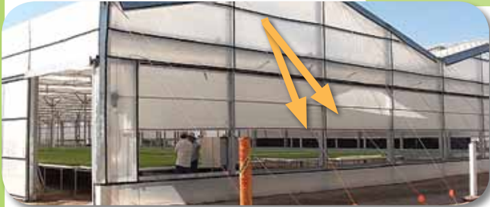
External cable bracing on the gable ends
