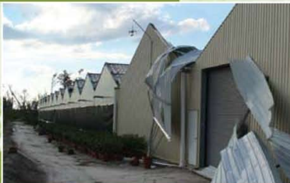
Non Cravo structures on right showing significant damage
